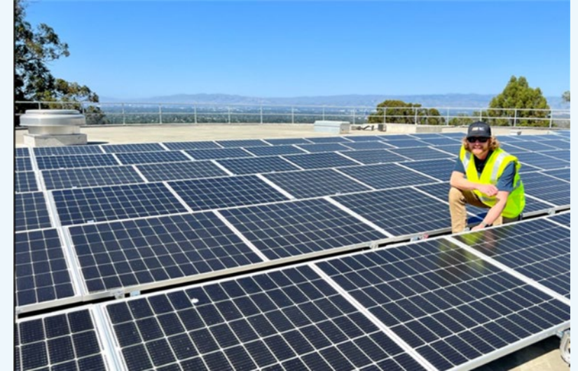
Solar generation at San Jose Water Company
