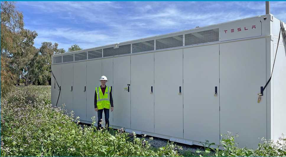
BESS on-site at San Jose Water Company's Williams Station
